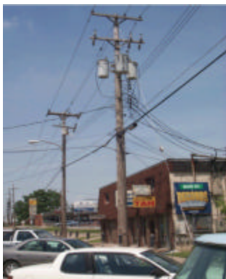
Figure 1.1 - A typical wooden class-4 (35 ft) utility pole
